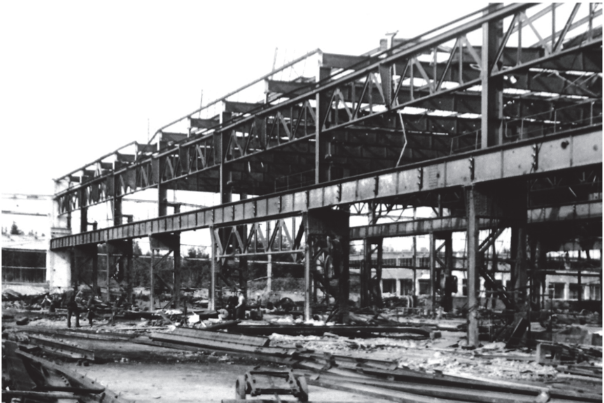
After Workshop V, it was the turn of Workshop VII to be completely dismantled. When this shot was taken, the ruins of Workshop VIII could still be seen in the right background. [Doku STV]
