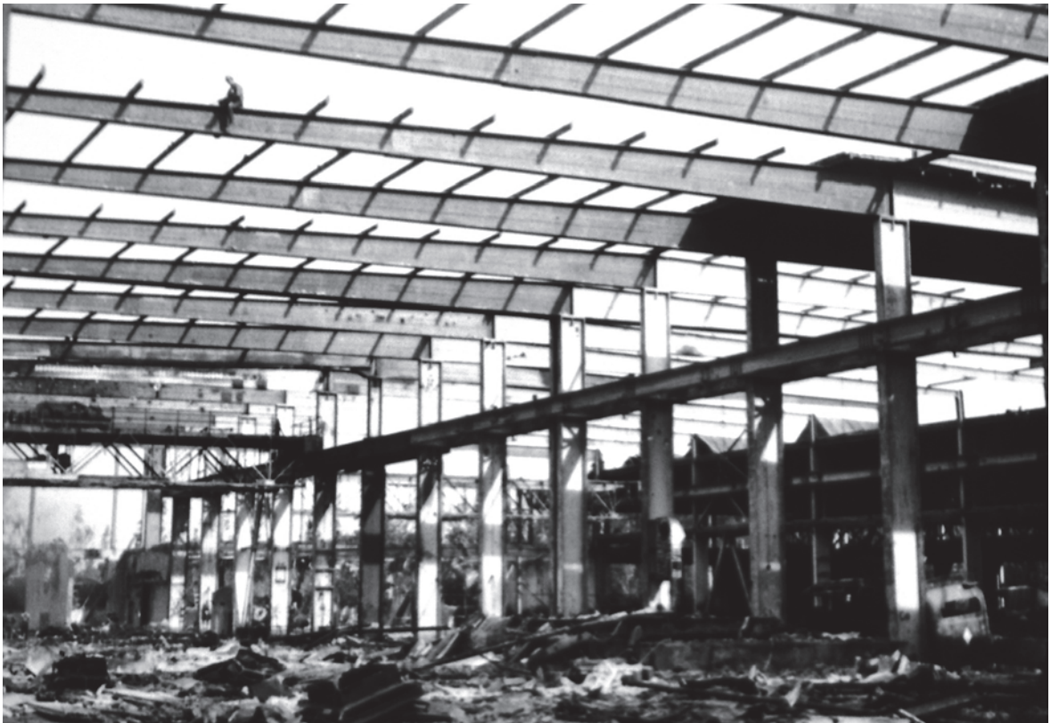
Following the removal of the machines and equipment as reparations, dismantling of Workshop V began. [Doku STV]
